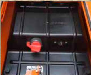
Battery cut-off switch
